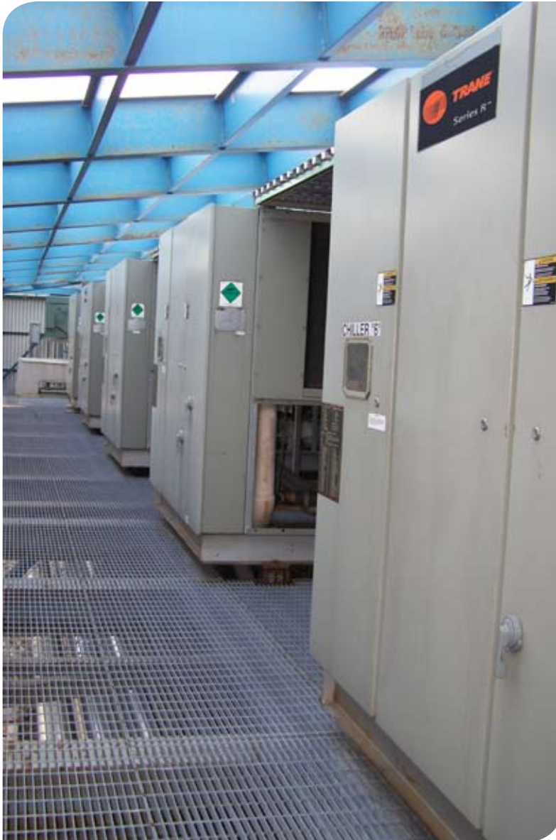
Trane air-cooled chillers installed at Savvis Communications' Weehawken, New Jersey, data center
